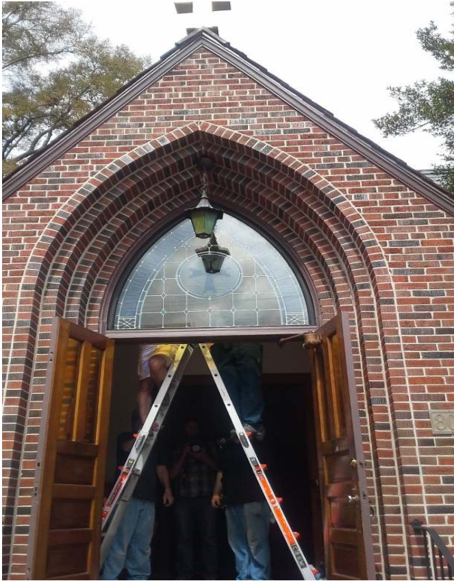
Leslie Miler, left, Paul Thornton and Gian Carlo, of C. Pickel Studio Inc., slowly raise a stained glass window into place at St. Michael the Archangel Church in Fayetteville, North Carolina.
